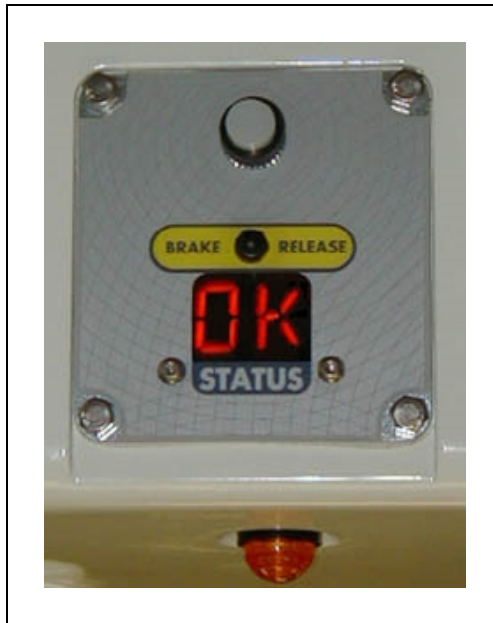
Figure 9-10. Status Display Panel, Showing 4 hex-head Bolts
